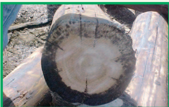
Creosote can leach from treated poles reducing its protection capability.
