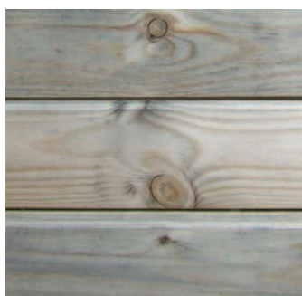
Untreated Pine cladding after just 9 months exposure displaying dark and unsightly staining.
