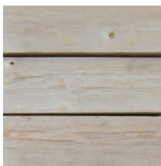
TANALISED Clear treated Pine cladding after 36 months exposure.
